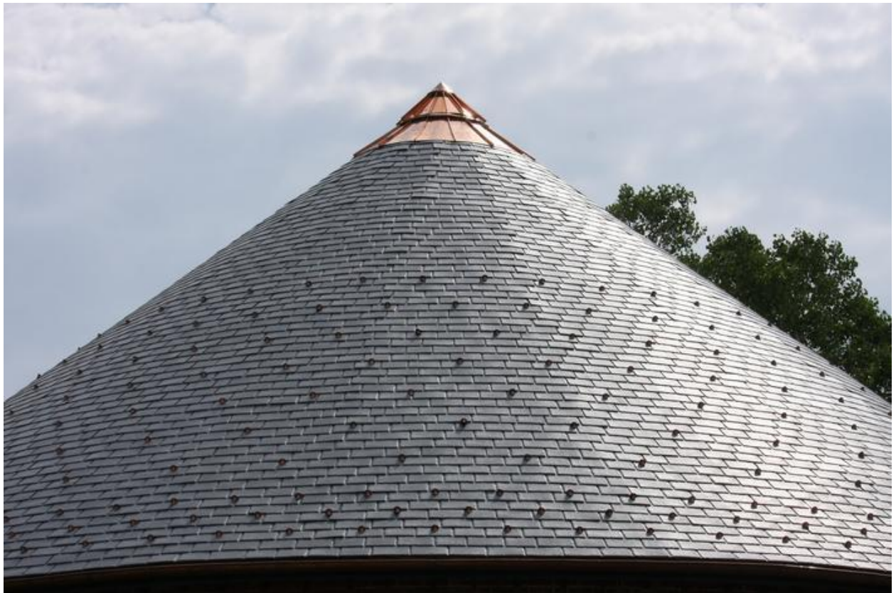
The first phase of the Gasholder Building renovation included restoring its distinctive circular dome.
