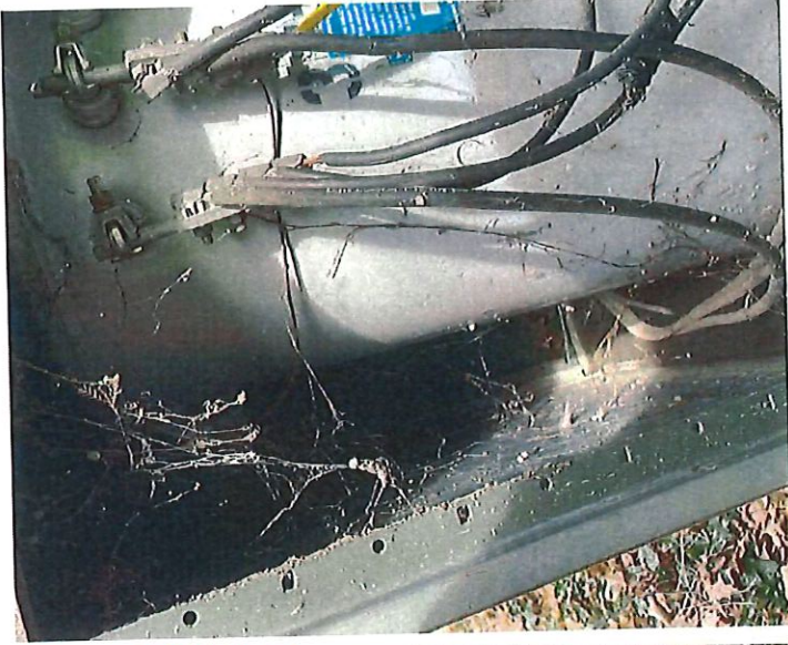
HAWTHORNE DR - REAR OF LOT #23 37 KVA TRANSFORMER & ENCLOSURE LV CABLES SOUTH SIDE OF ENCLOSURE
