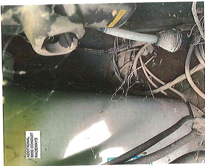
HAWTHORNE DR - REAR OF COLONY LOT #23 37 KVA TRANSFORMER & ENCLOSURE MV & LV CABLES SOUTH SIDE OF ENCLOSURE
