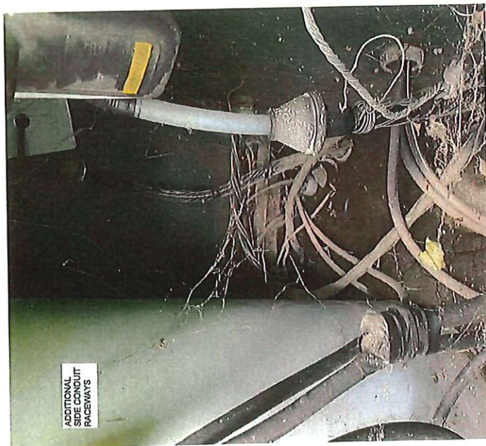
HAWTHORNE DR - REAR OF COLONY LOT #23 37 KVA TRANSFORMER & ENCLOSURE MV & LV CABLES SOUTH SIDE OF ENCLOSURE
