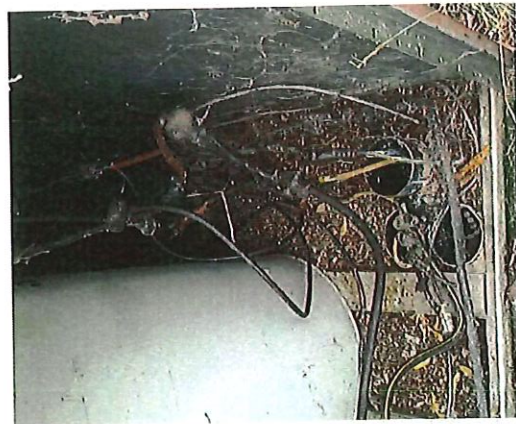
HAWTHORNE LOT 19 37 KVA TRANSFORMER
