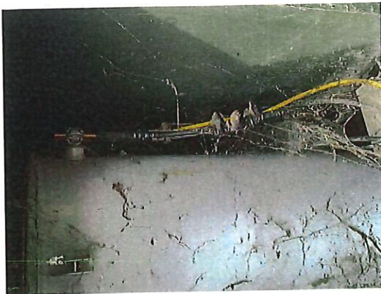
HAWTHORNE LOT 19 37 KVA TRANSFORMER
