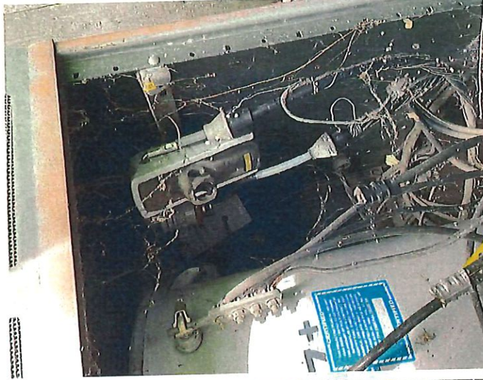
HAWTHORNE DR - REAR OF COLONY LOT #23 37 KVA TRANSFORMER & ENCLOSURE MV & LV CABLES SOUTH SIDE OF ENCLOSURE
