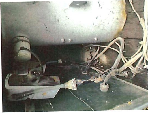
HAWTHORNE LOT 19 37 KVA TRANSFORMER
