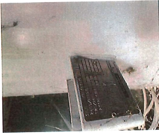
HAWTHORNE LOT 19 37 KVA TRANSFORMER
