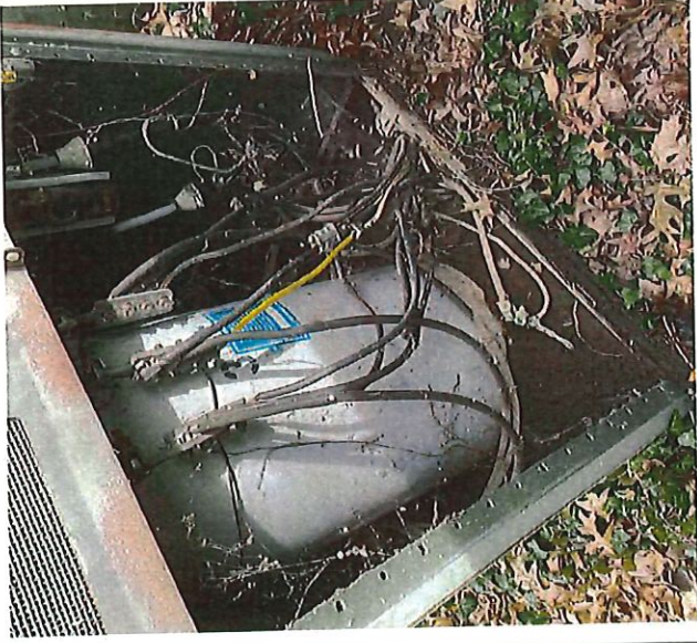
HAWTHORNE DR - REAR OF LOT #23 37 KVA TRANSFORMER & ENCLOSURE MV & LV CABLES SOUTH SIDE OF ENCLOSURE
