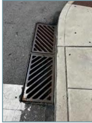
Figure 10: Graphic showing a storm drain incompatible with bike-safe design, as bike tires could fall into slots of storm drain, causing injury.
